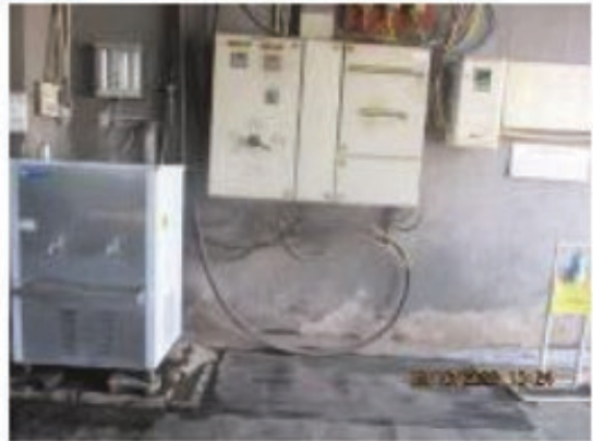
Water around rubber mat near electrical panel.JPG
