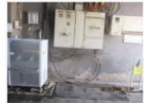
Water around rubber mat near electrical panel.JPG
