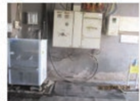
Water around rubber mat near electrical panel.JPG
